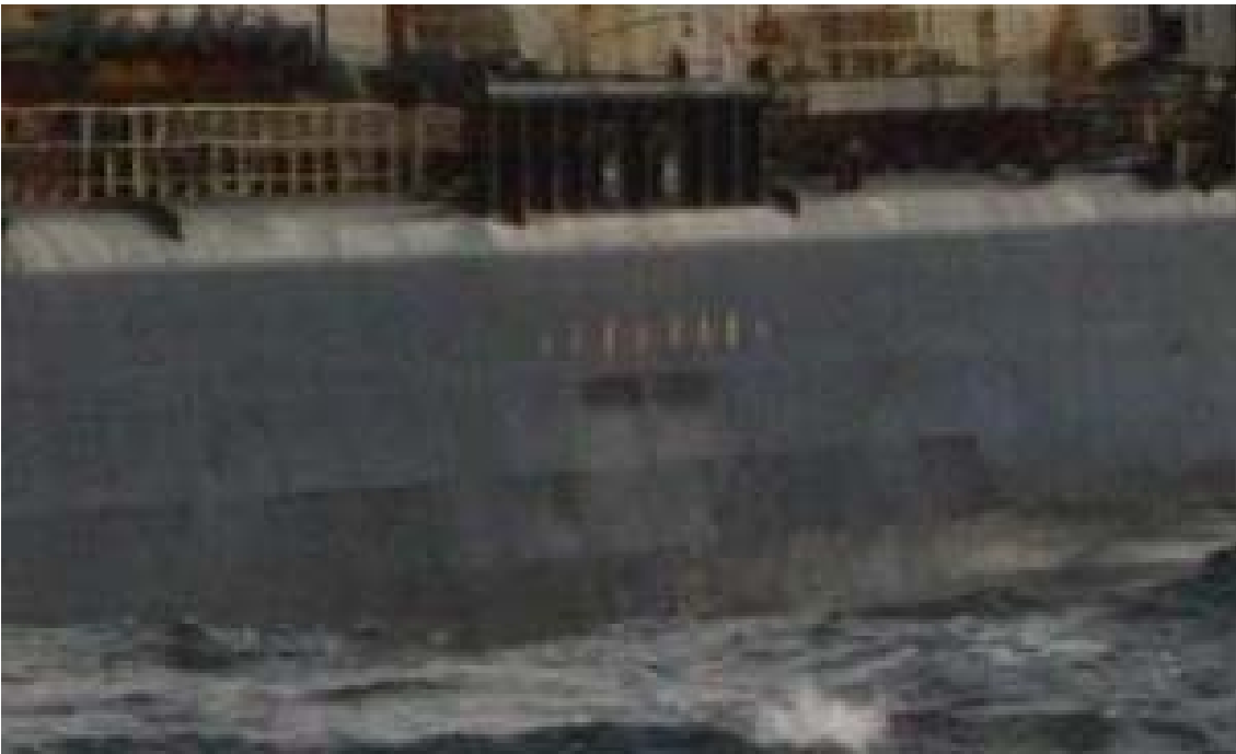
Setting in of shell plating beneath hose rack on port side of the vessel (Between frames 67 and 69)
