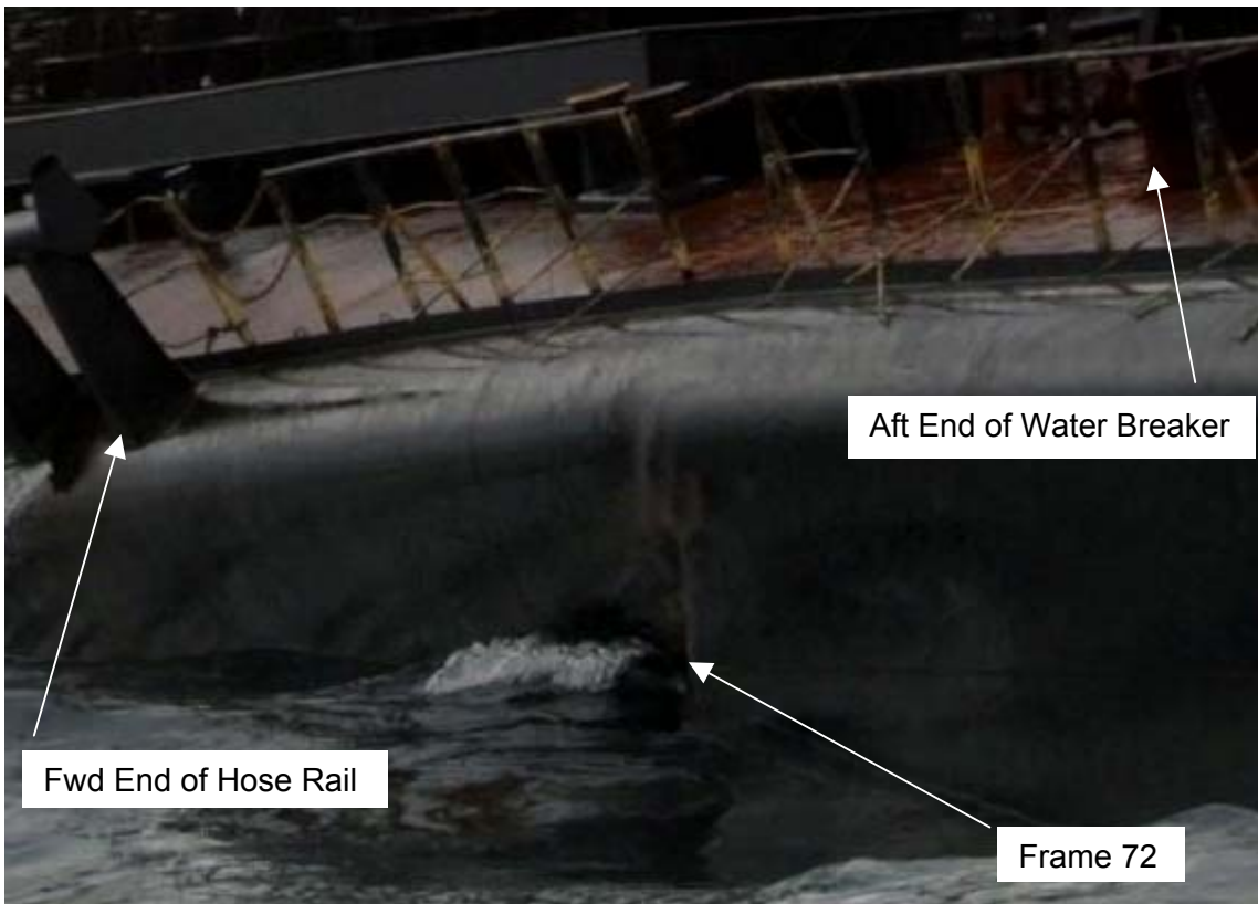
Forward most deformation of main deck edge and side in way of 3 Starboard Ballast Tank and 2 Starboard after wing tank
