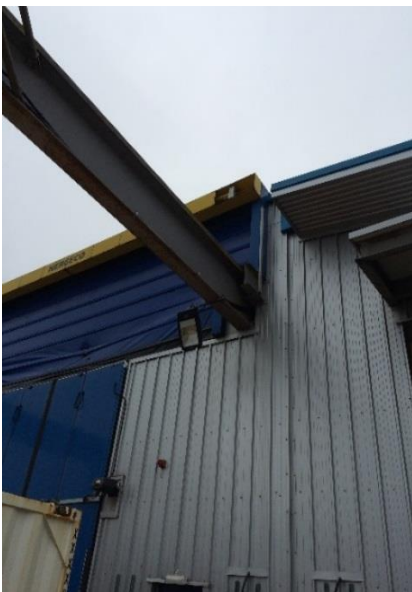
Item dropped approximately 7-10 meters from above the main roller shutter door
