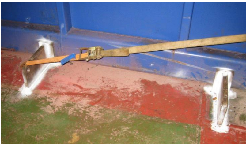
The above figure shows Welds on 'no hot-work' zones
