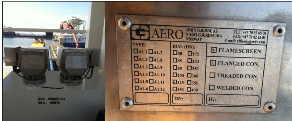
Photo 4 - Fuel Oil Overflow Vent (Typical)
