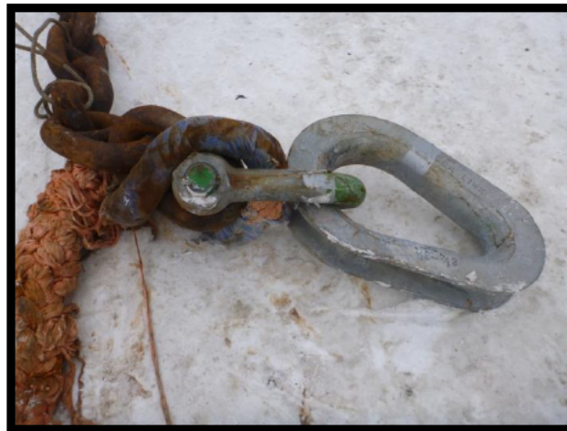
Figure 75: Photo of recovered emergency towline (eye on the KULLUK end of the emergency towline) showing missing thimble lashings allowing towline to separate from hard thimble. Blue Cordura® protection is also damaged. ( USCG Photo )
