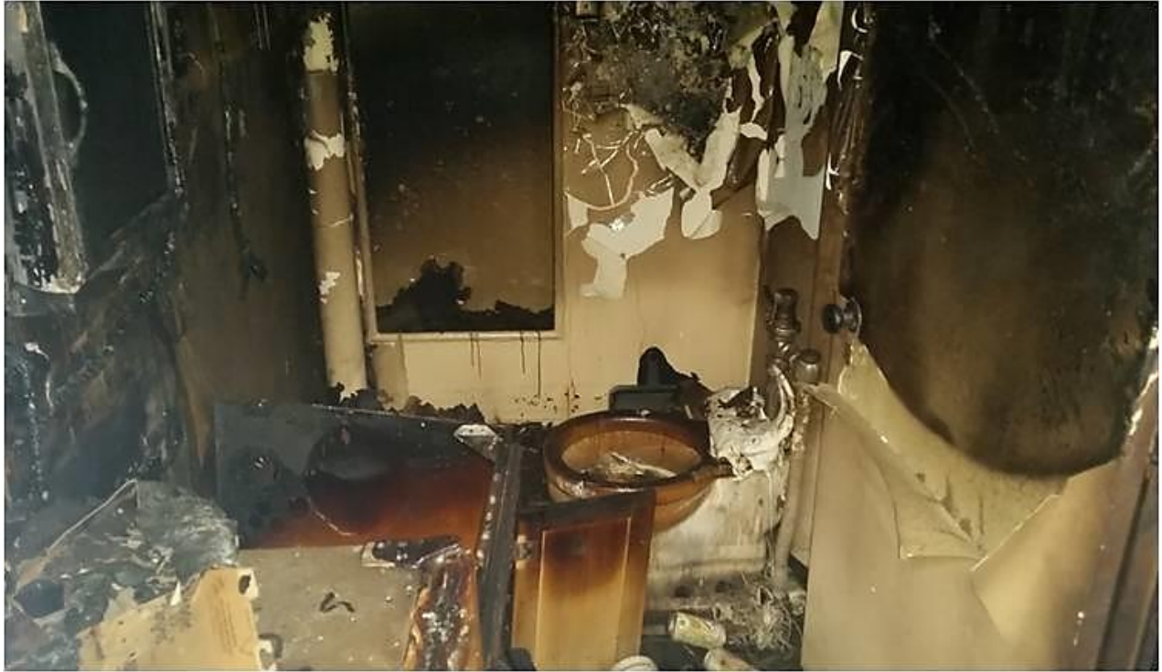
Fire damage to one of the Alpena bathrooms. (Photo by Coast Guard)
