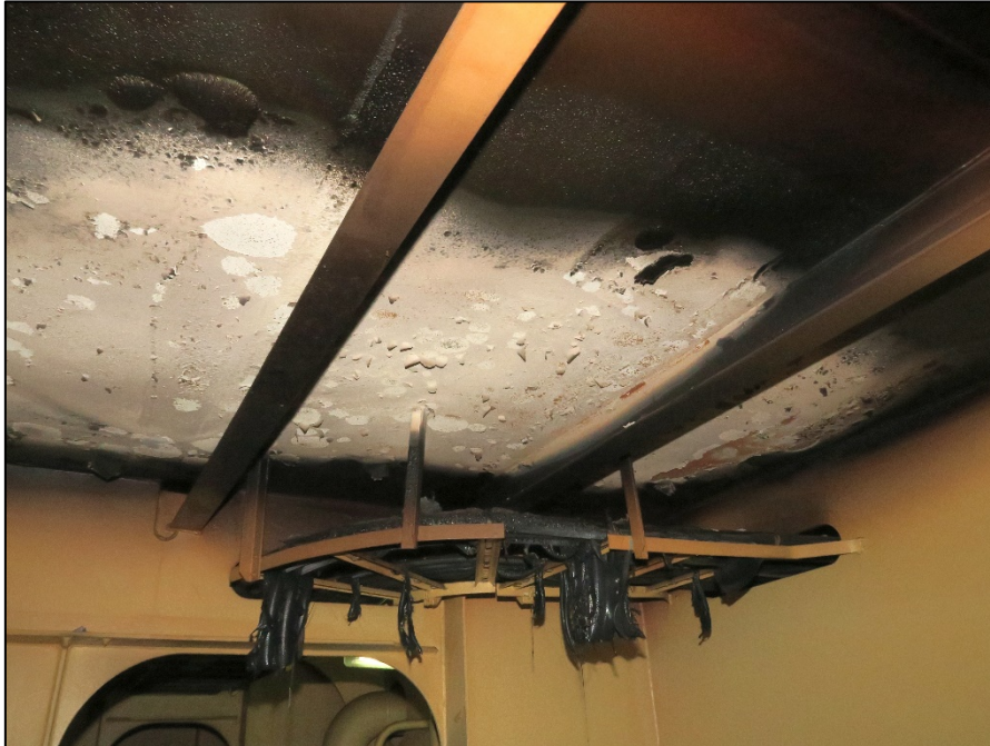
Figure 25: Thermal damage in the starboard passageway adjacent to bay 3
