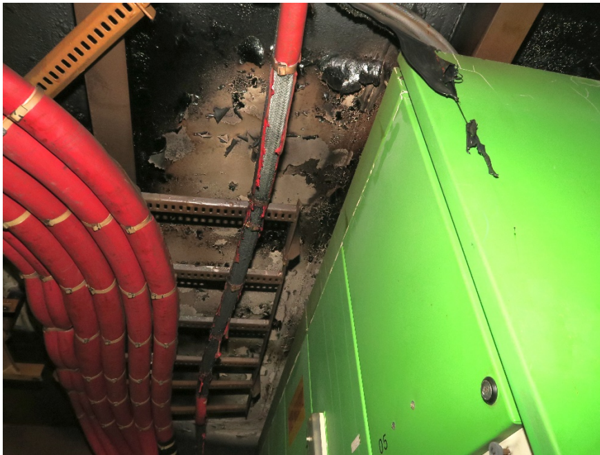
Figure 27: Thermal damage in the starboard passageway adjacent to bay 7
