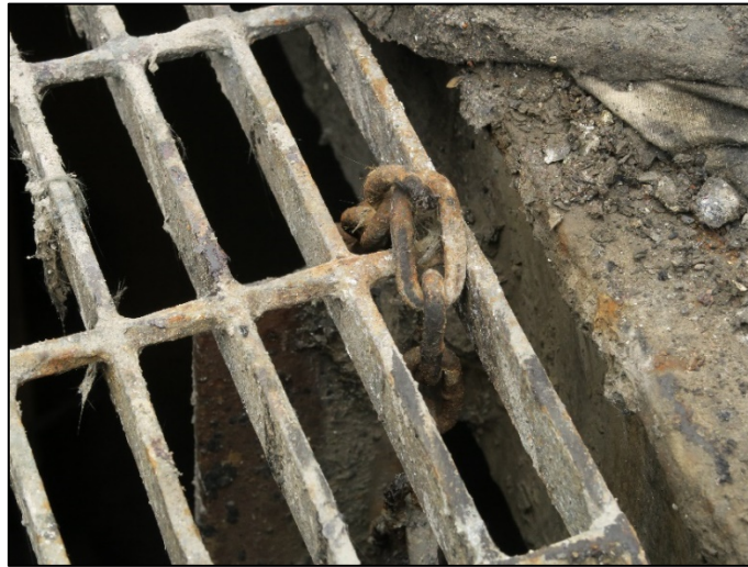
Figure 55: Grill over ventilation opening secured by chain and lock
