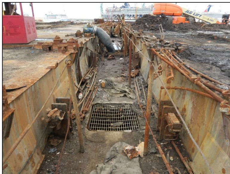
Figure 54: Grill over port ventilation opening in the transverse corridor between bays 4 and 8
