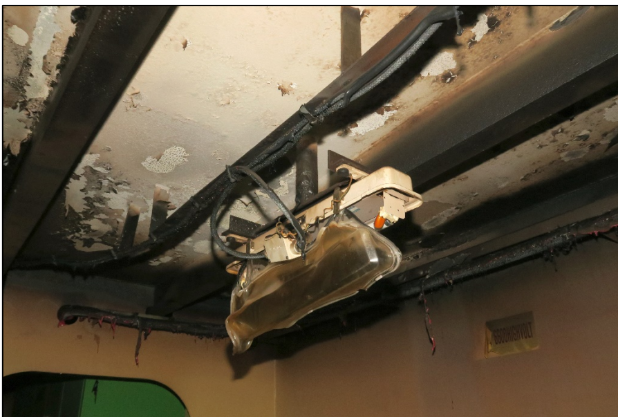
Figure 26: Thermal damage in the starboard passageway adjacent to bay 5
