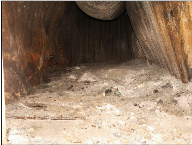
Figure 30: View into the container at slot 120582 Small amount of fire debris; floor completely burnt.
