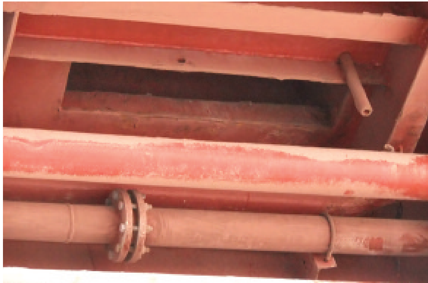
Ventilator opening in deck at the aft bulkhead of cargo hold No. 3. The steel bulkhead is the common boundary between the accommodation and the cargo hold ventilator.
