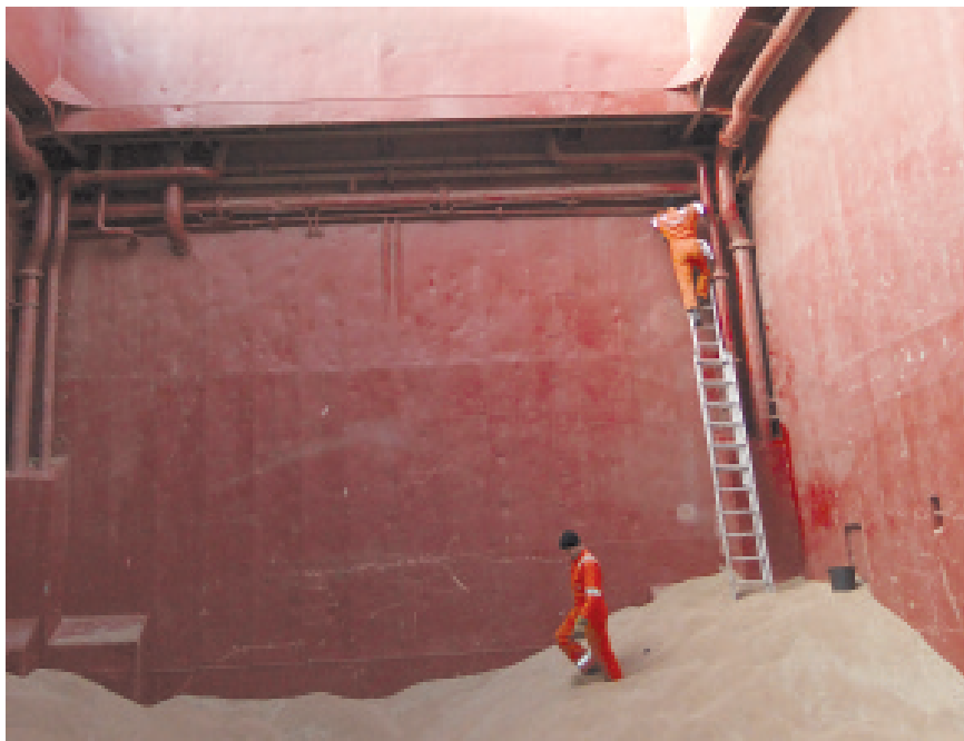
Aft bulkhead of cargo hold No. 3. The ventilator opening is in the corner, above the ladder. Access is difficult, as it is behind pipes under deck.
