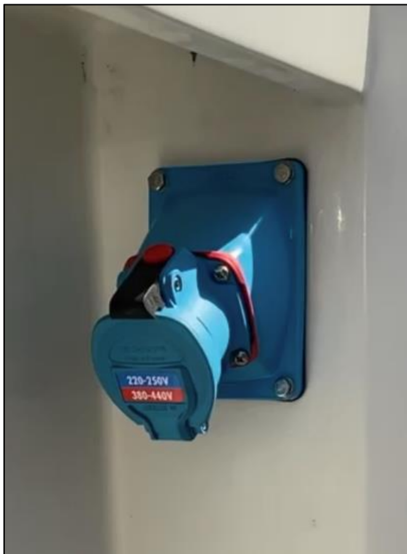
Figure 3: Water scooter charging socket (fitted by the crew members in June 2021)
