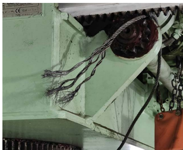
Figure 1: Failed crane hoisting wire
