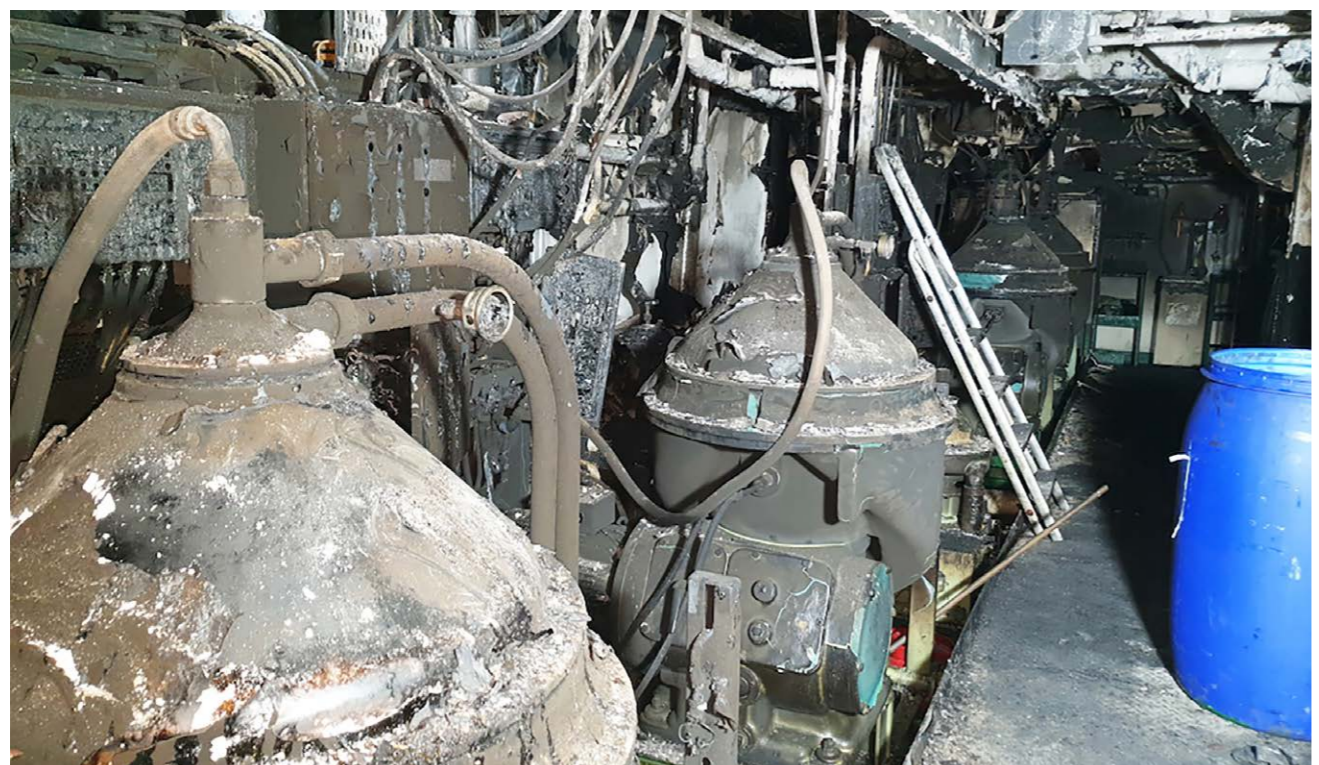
Figure 1: Fire-damaged fuel purifier room
