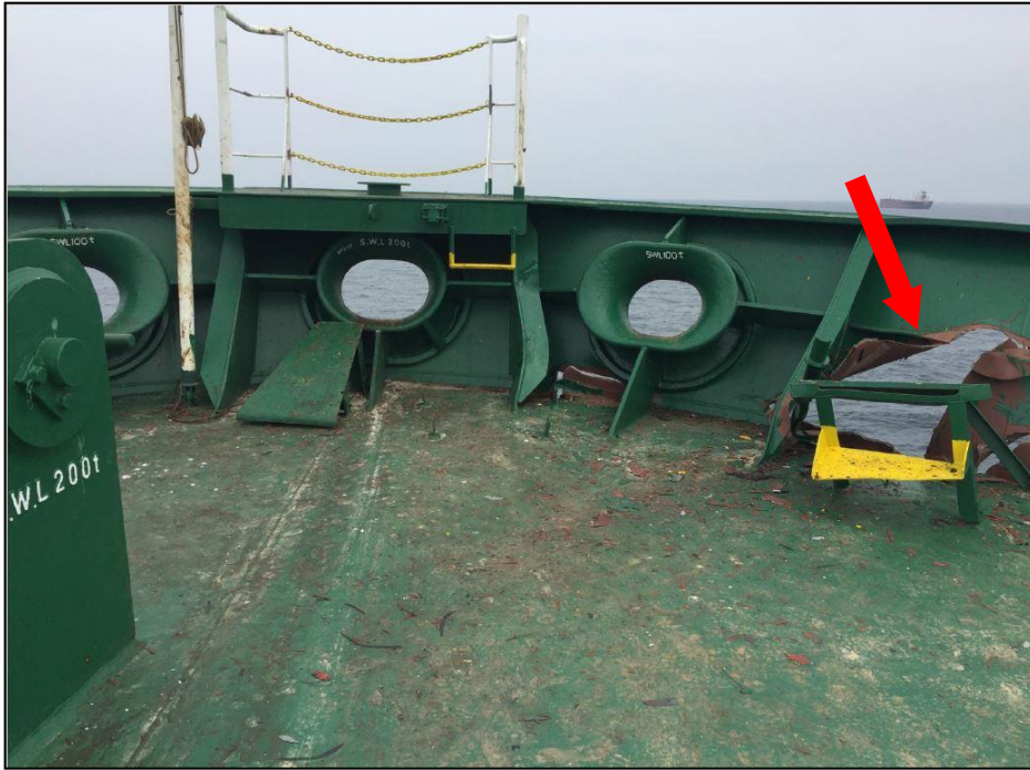
Figure 19: Damaged bulwark and stiffeners on the forecastle
