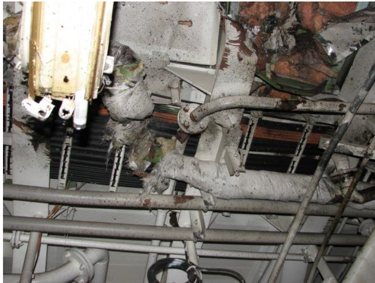
Figure 5. One area of damaged overhead/piping caused by a flywheel fragment
